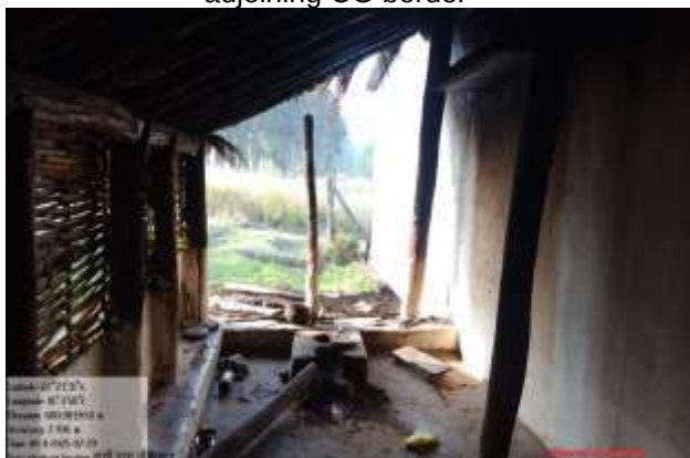
Village hut kitchen damaged by Elephant
